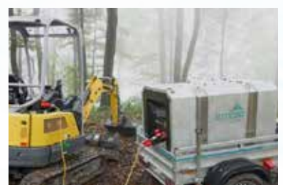
Axpo Butler S A plug-and-play solution for the rapid provision of electricity to remote sites.
